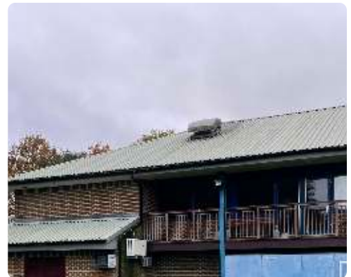
Water ingress was apparent throughout the building. Additionally, due to poorly performing insulation the building was proving costly to keep warm during the cold winter months.
