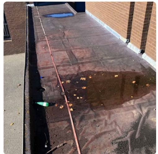
Existing waterproofing system and the overlaid bituminous membrane were failing in places
