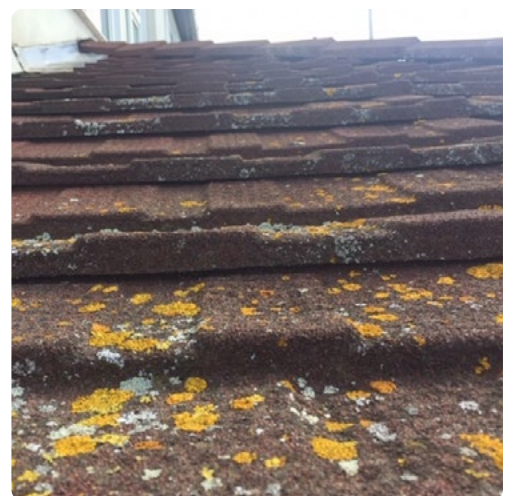
Pitched sections were beginning to display significant failures
