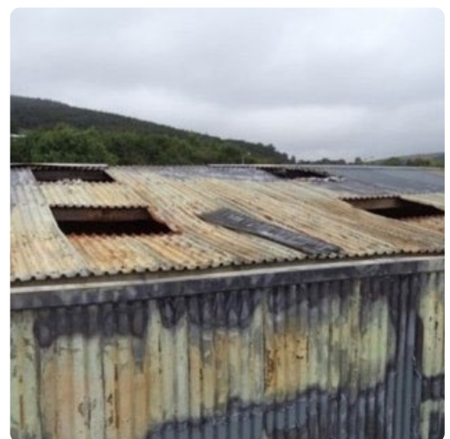
Building damage and poor condition of the existing roof sections and walls
